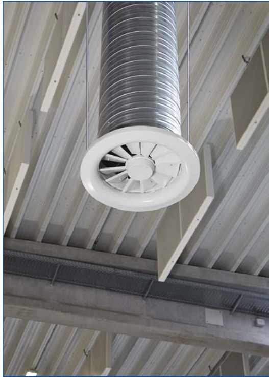
Freely suspended installation
