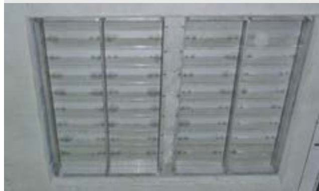
Ceiling damper unit on the driving side
