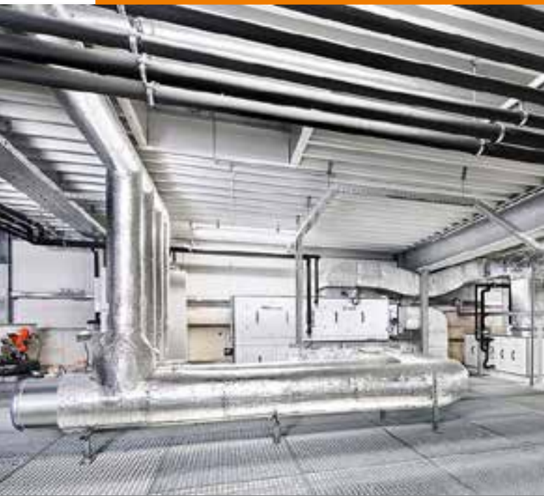
The plant room in the TROX administration building.
